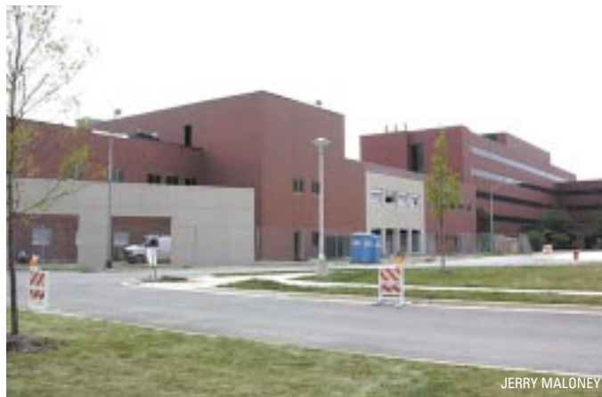
The new 34-bed blind rehabilitation center now under construction at the Hines VA Hospital is expected to be completed in late fall.
