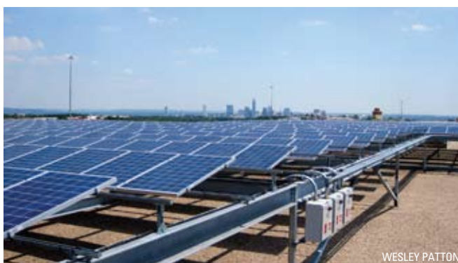
The Austin data center installed a 15,000-square-foot rooftop solar array.
