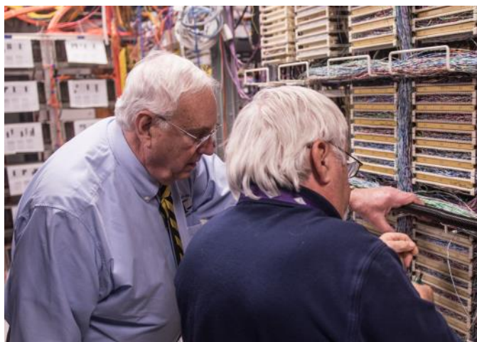
Above: SCI Founder and CEO John P. Molière and team member Jim Davis execute telecommunications services in a VAMC Switchroom
